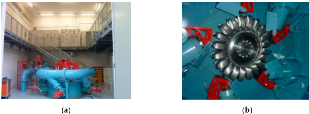
Figure 36. Mini-hydropower plant with Pelton turbine connected with Permanent Magnet Generator: (a) Picture of the entire hydropower plant; (b) Specific of Pelton turbine with the vertical axis of rotation and six jets.
